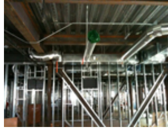
Typical duct run with a bit of creative coordination to make the structural beam “disappear.”
