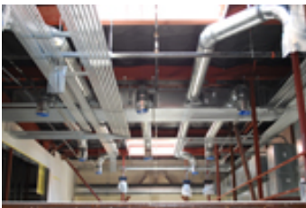
Theater ductwork illustrates the tight coordination required with structural, electrical, and fire/life safety. As part of the CHPS program, all duct openings must be kept wrapped and sealed during every stage
