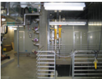
Air handling units were fitted into the limited space required (120" X 36") leaving only 3 inches from the top of the duct to the slab above.
